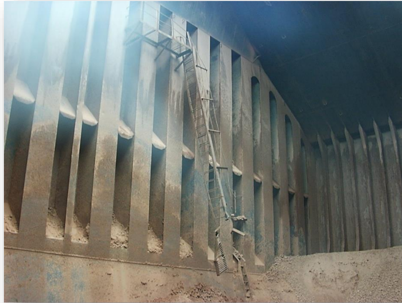
Hold access ladders may become damaged
