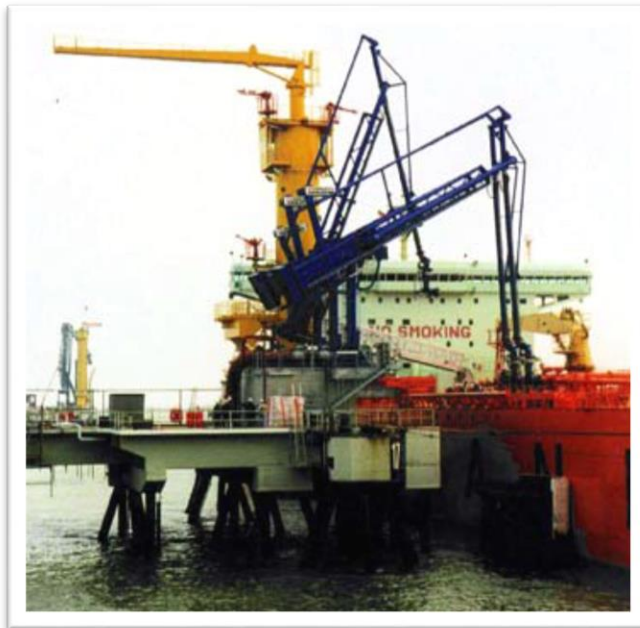
Photograph showing a typical view of a transfer of bulk liquids or gas using fixed arms
