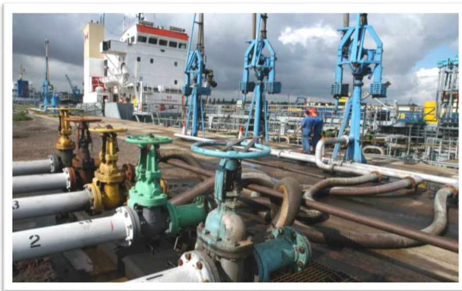
Typical illustration of slips and trips hazards on a bulk transfer jetty installation using fixed arms and flexible hoses
